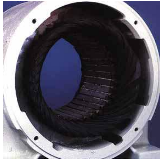
#10 Damage Due To Overload
